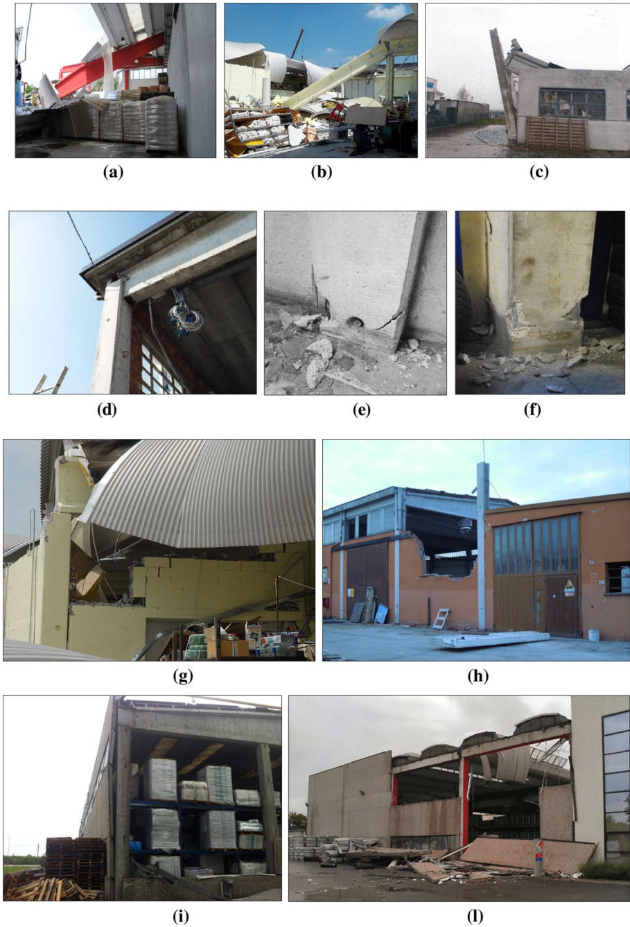
Fig. 6 Collapse and damage mechanisms observed in the buildings of the case-study area of San Felice
