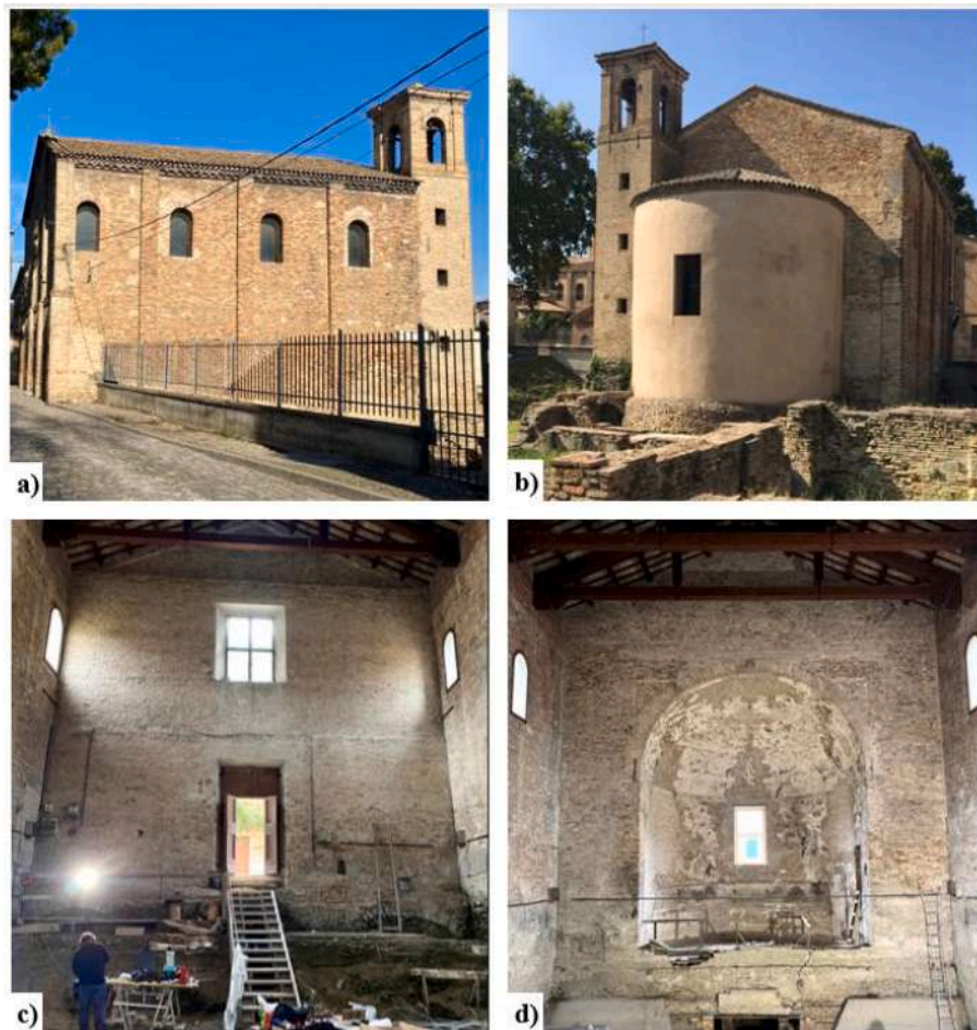
Fig. 3. The church of Santa Croce in Ravenna: a) exterior - south façade; b) exterior – east façade and apse; c) interior – main façade (west wall) and entrance; d) interior – east wall and apse.
