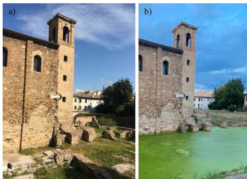
Fig. 1. a) the church of santa croce in September 2020 (south wall with bell tower), with the surrounding archaeologic area; b) the same zone during the flooding due to the pumping system failure in August 2021.
