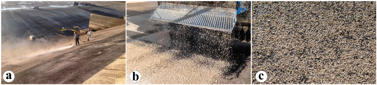
Fig. 3. a) High pressure cleaning and resealing of the embankment surface; b) Application of an in-situ sealing membrane; c) Multi-layered in-situ sealing membrane with aggregate finishing.
