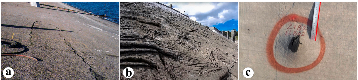
Fig. 2. Common failures on asphalt dams: a) Cracking failure (Los Angeles, USA) [21]; b) Slippage failure (Paduli, Italy); c) Blistering failure (Zhangewan, China) [10].
