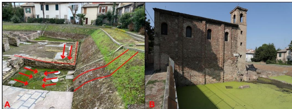
Fig. 5. A) Evidences of the ground settlements and of the slope instability in close proximity of the tank. B) View of the archaeological site entirely flooded during the pump break down in August 2021.
