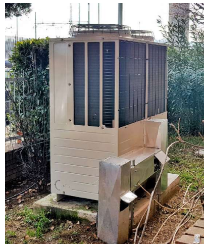
Figure 1: CO 2 heat pump installed in the flat complex.
