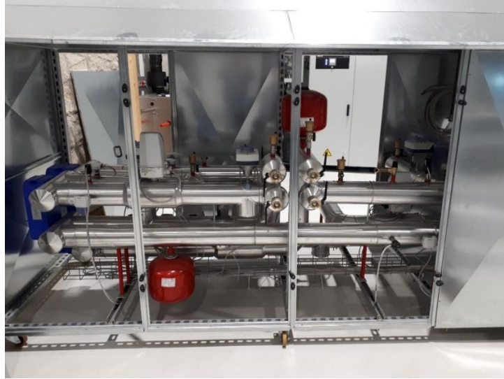
Figure 3. Inside of the prosumer substation.
