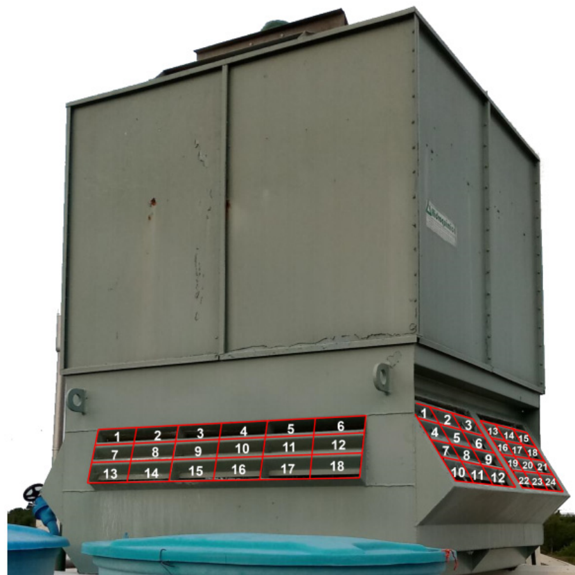
Figure 2. Divisions of the air intakes of the industrial refrigeration unit of the evaporative condenser for the measurements of the inlet velocity.
