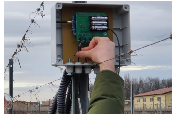
Fig. 7. A LoRaWAN low power multi-sensor node installed in the Italian pilot
