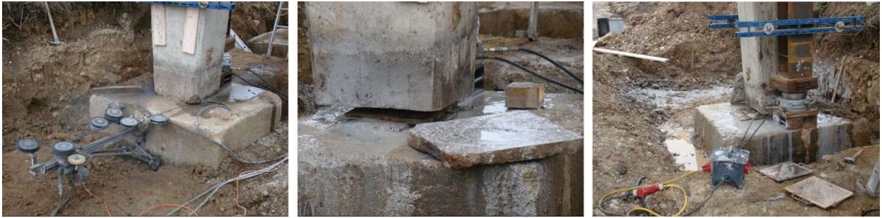
Fig. 7: Photographic documentation of the pier settlement process [72].
