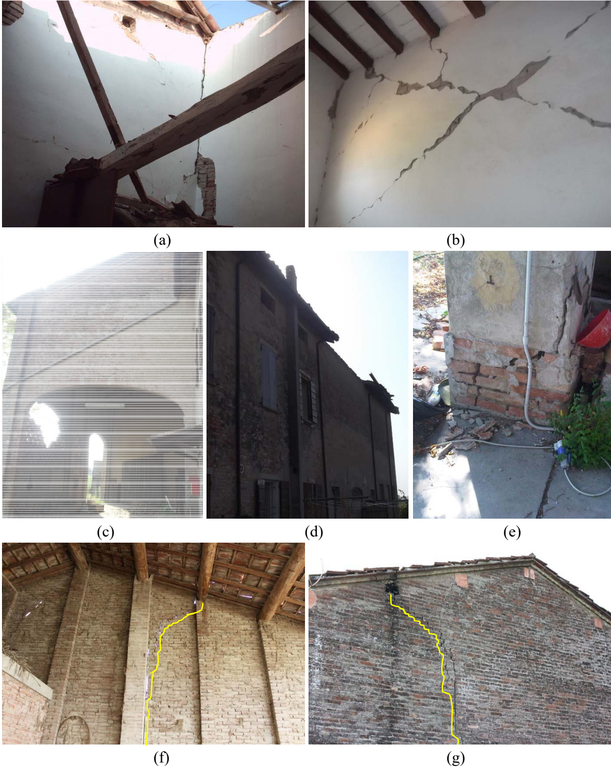
Figure 16. Detail of damage to category B buildings and non-structural elements. (a) Fall of timber roof beams from the intermediate wall in the composed bldg. # 8. (b) Shear cracks on a wall (bldg. #8). (c) Failure of “gelosie”, typical holed infill walls (bldg. #5). (d) Fall of a portion of the perimeter masonry cornice (bldg. #5). (e) Cracking at the base of a masonry column portico (bldg. #7); (f) Internal and (g) external view of the detachment of the infill panels from the bearing columns due to a poor connection (bldg. #12).
