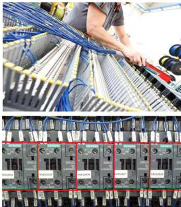
Fig. 5. Different views of a switchgear during the assembly. The cables and components, often very similar and of the same color, make complex the detection of a specific terminal or wire from the scene.
