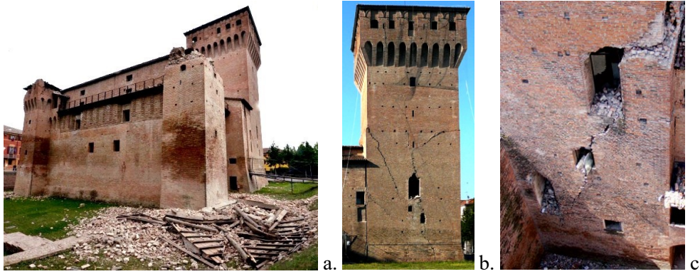
Fig. 4 - San Felice sul Panaro fortress after the Emilia Earthquake (2012): (a) collapse of the minor towers' crowning, main tower's South front (b) and North front (c).
