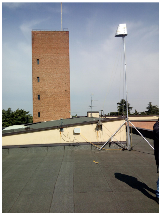
Figure 3. The installation of a thermal camera in a fixed position for the continuous monitoring of surface temperature.
