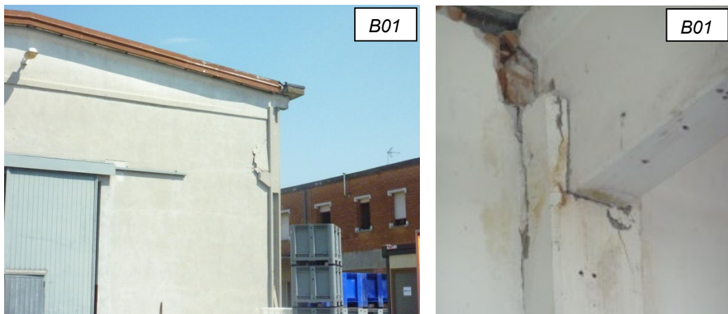
Figure 10. (a) Precast RC building with regular masonry cladding walls, only slightly damaged by the earthquake; (b) Damage to the column fork, due to the transverse rotation of the double slope roof beam during the ground motion.
