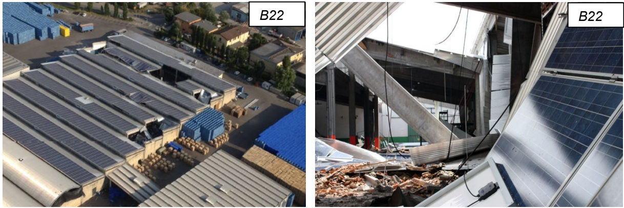
Figure 21: Collapses in a recent fruit warehouse with inclined precast beams to realize a shed structure.
