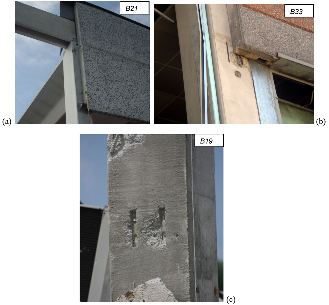
Figure 29. Damage of fastening devices for panel- column connections when their deformation capacity was exceeded.
