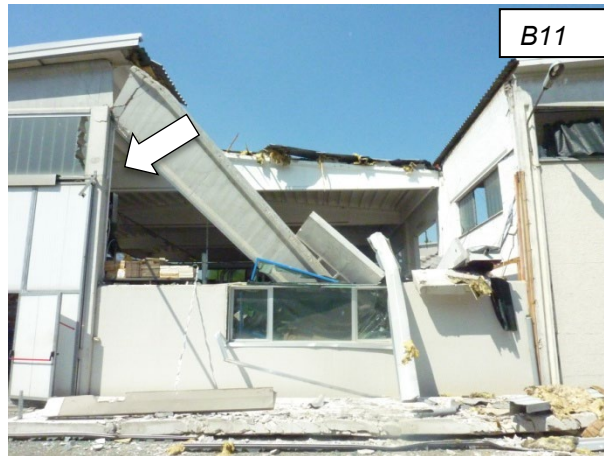
Figure 15. Collapse of the beam of the facade frame due to the interaction with the non structural columns indicated with an arrow.
