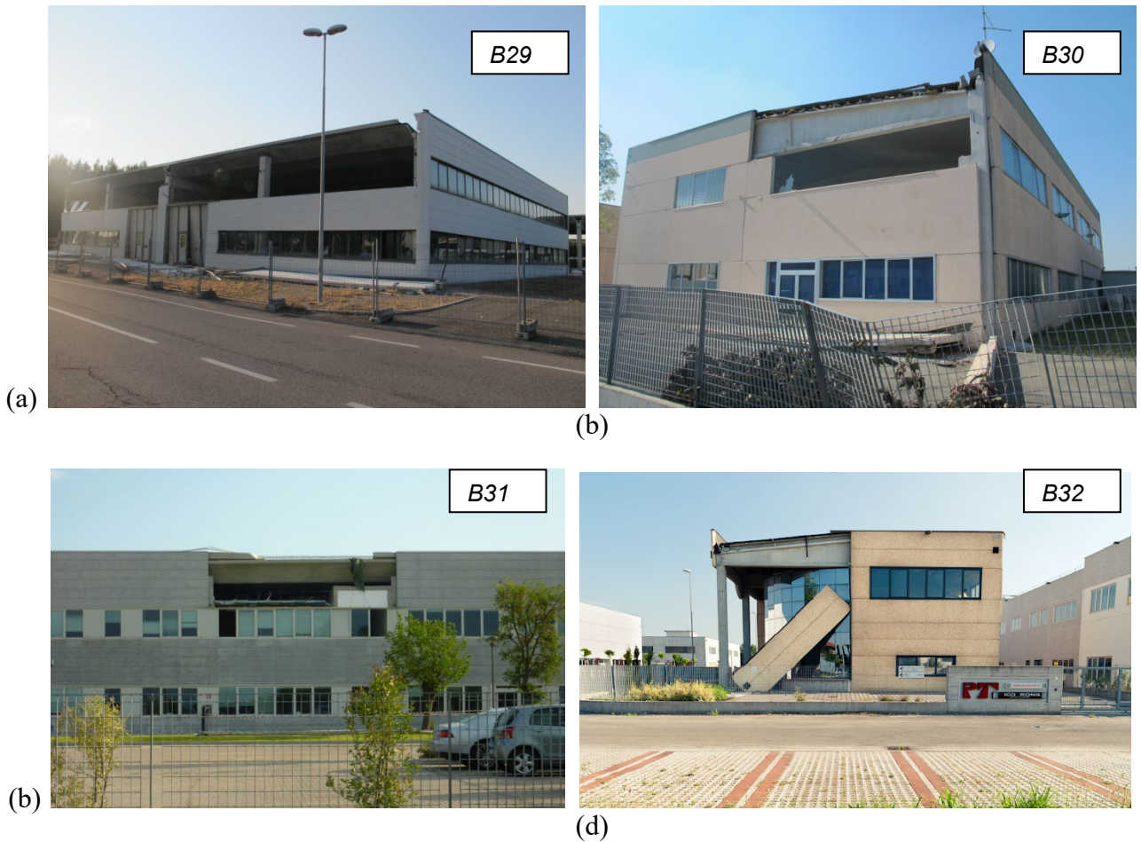
Figure 28. (a – d) Collapse of horizontal precast cladding panels.
