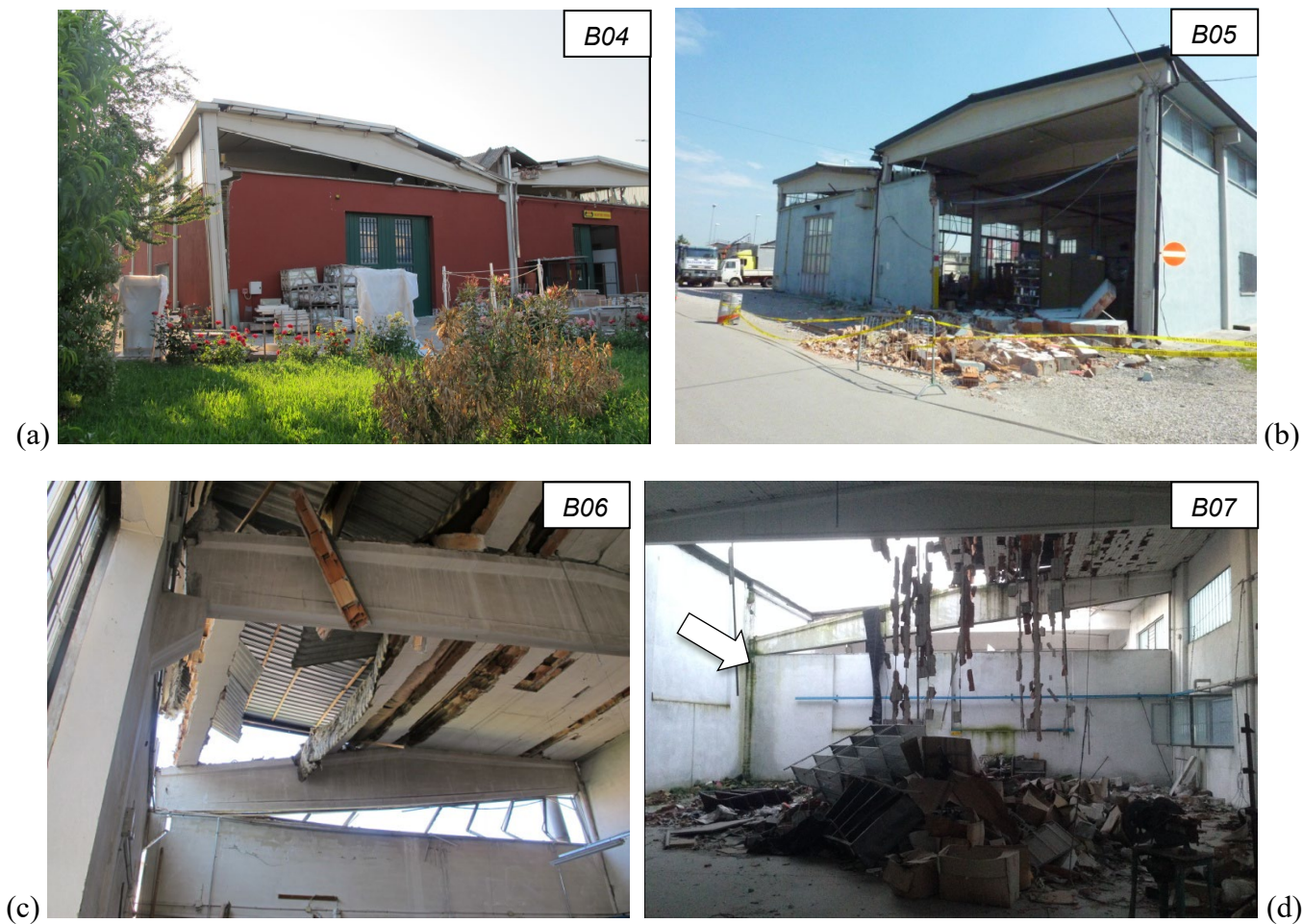
Figure 12: (a, b, c) Collapses due to the presence of strip windows on the top of masonry walls (the building in picture (a) is the same shown in Figure 7b before the collapse); (d) collapse due to the presence of an internal masonry wall (indicated by an arrow).
