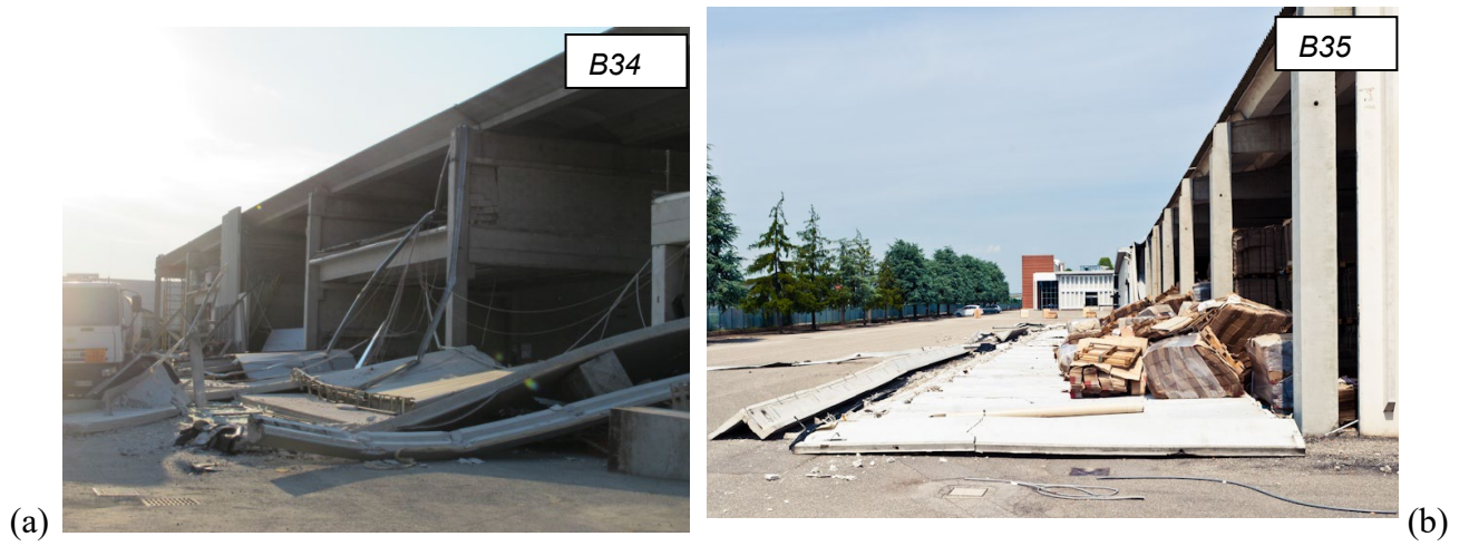
Figure 30. Collapse of precast cladding panels non properly restrained at the base.
