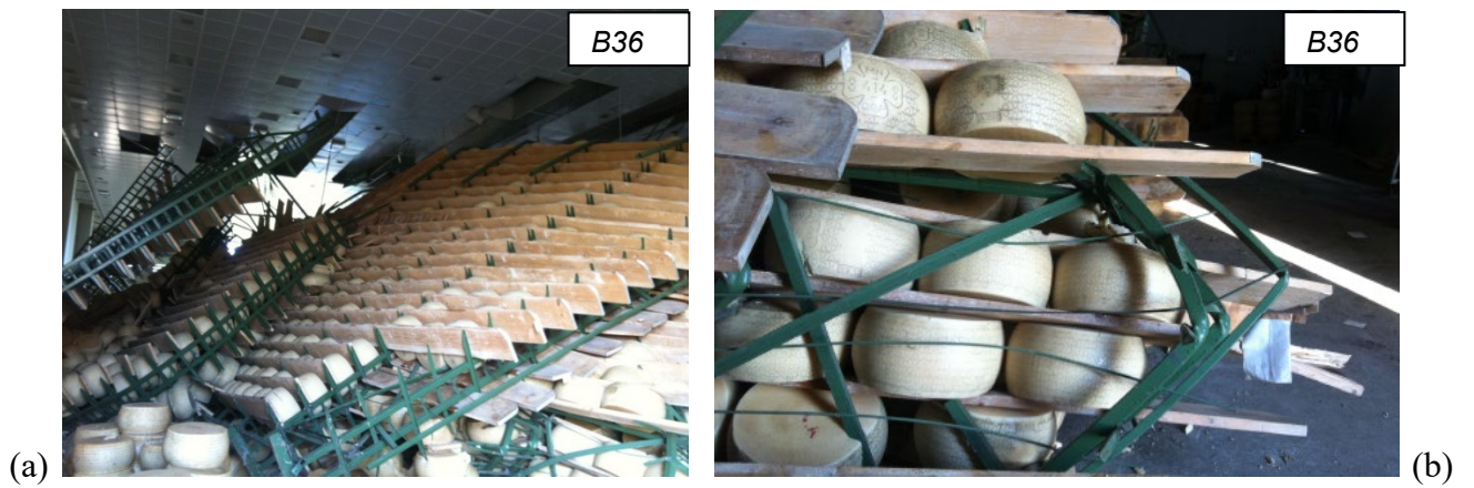
Figure 31. (a) Collapse of a cheese warehouse in the province of Mantova, (b) detail of the light steel structure made of cold-formed steel profiles not designed to bear horizontal loads.
