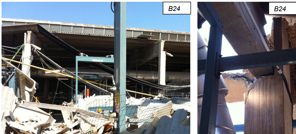
Figure 23. Complete collapse of an industrial building due to lateral overturning of beams.
