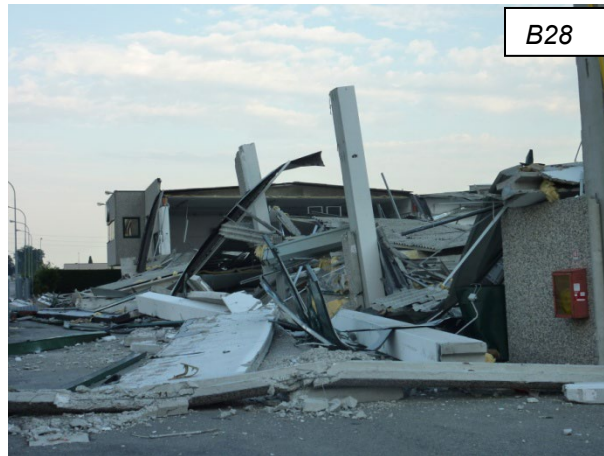
Figure 27. Complete collapses of an industrial building in S. Agostino, with large base rotations of the columns probably due to rotation of foundations.
