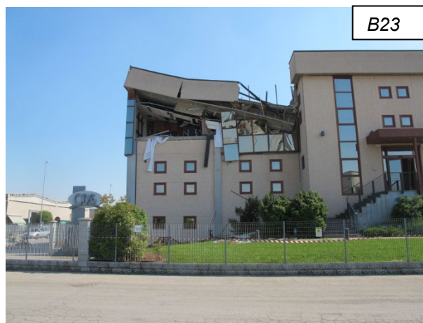
Figure 22. Failure due to the loss of support of roof elements related to plan-irregularity a commercial prefabricated building.
