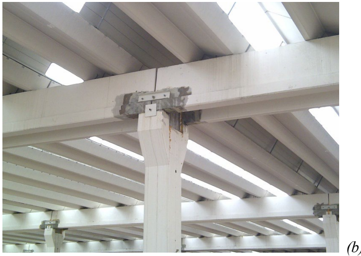
Figure 8. (a) Precast buildings with planar roof (Type 2) and (b) long prestressed omega-shaped girders with thin-web roof elements for a production area. In the picture, the detail of a safety intervention executed before restart the working activity is also shown.
