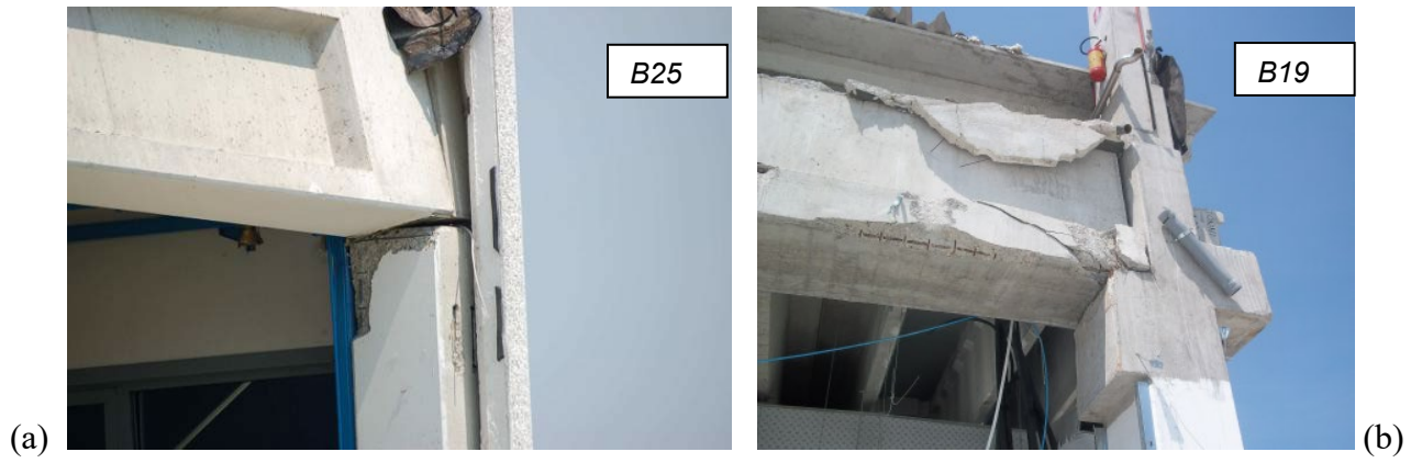
Figure 24. (a, b) Permanent lateral beam rotations in two partially collapsed buildings.
