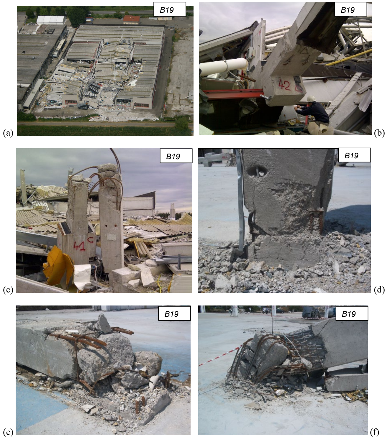
Figure 26. A collapsed building in Cavezzo (MO): (a) Aerial view, (b) column rotation due to the formation of a flexural plastic hinge, (c) rupture of a column in an intermediate position due to the presence of a TT precast slab, (d) plastic hinge with bar instability, (e) flexural failure with bar necking, (f) shear failure of a highly reinforced column in flexure.
