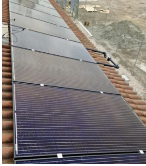
Figure 4: PVT system on the roof
