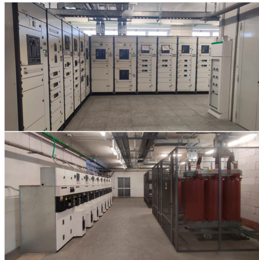
Figure 2. Picture from the LV and MV substations in the building.
