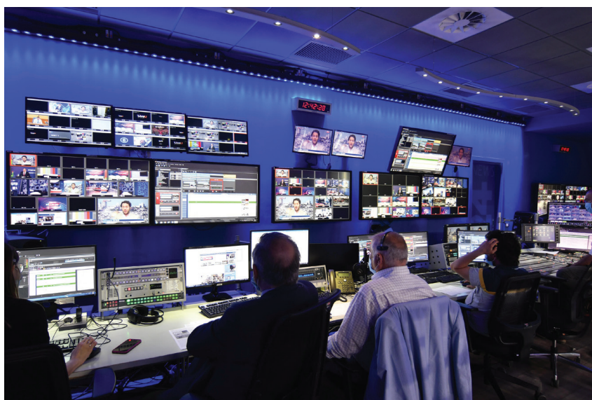
Figure 4. Control room at Mediaset's Production Centre in Cologno Monzese (Milan) (courtesy of Mediaset Press Office).
